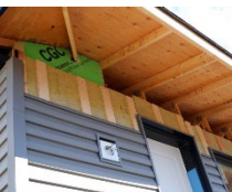
* Thermafiber Rainbarrier HC ci mineral fiber insulation and strapping below vinyl cladding
