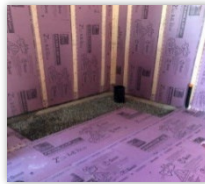
*Radon abatement system
