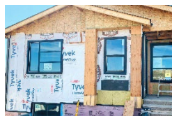
* Below grade to exterior insulation transition using Foamular C200 and Rainbarrier HC ci
